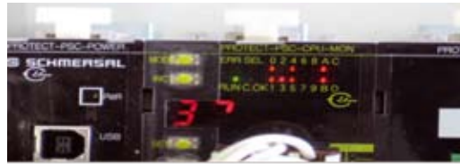
Fig. 9: Clear display on the CPU module of which input and output signals connected
